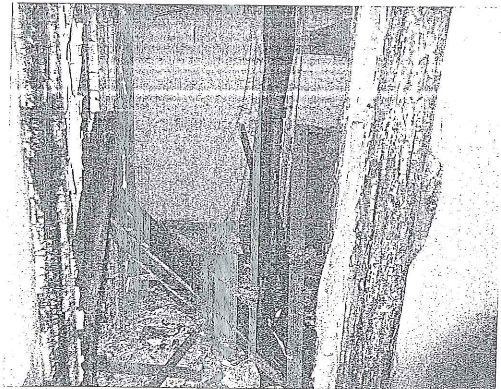
INTERIOR VIEWS INDICATING TYPICAL POOR CONDITION
