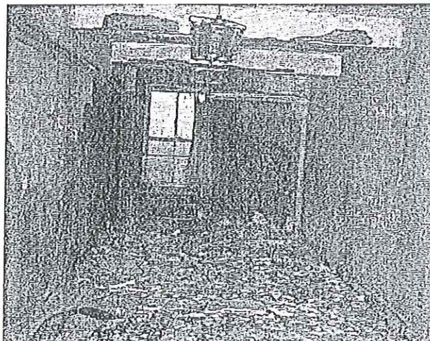
Photo 15: The finishes and concrete slab at the southwest corner of the building are saturated at the upper floors. The areas of saturation are smaller on lower floors, but are generally still present. Continued exposure to water will, ultimately, lead to corrosion of the steel reinforcing in the concrete, corrosion of the steel frame, and a reduction in the capacity of the structure to carry load. Freeze-thaw damage may also occur as the building is unoccupied and unheated
