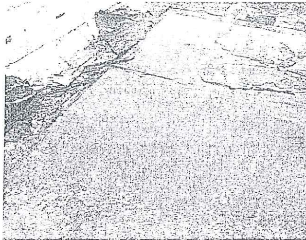
Photo 16: The roof membrane is missing and the roof drain is plugged at the southwest corner of the roof at the Nelson House Annex. This condition will lead to deterioration of the concrete and steel frame (see caption for Photo 15). In the near term, the plugged drain may lead to accumulation of water and/or snow on the roof that will exceed the capacity of the concrete or steel structure, leading to a local collapse of the roof.
