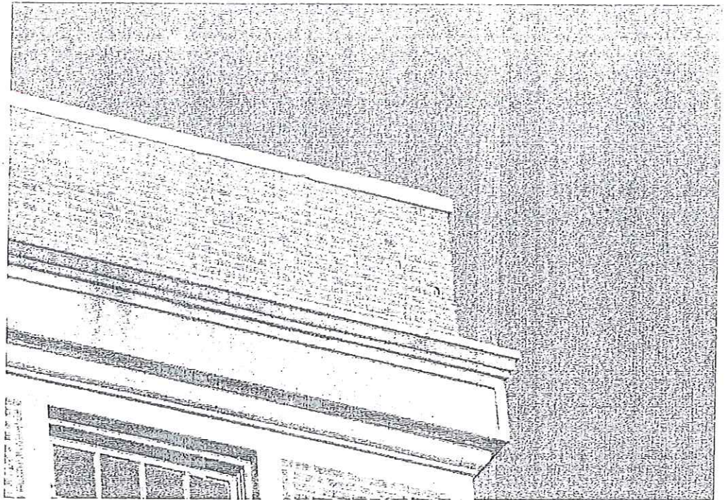
MASONRY CRACKS AT PARAPET
