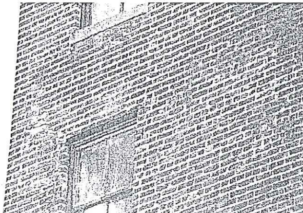
Photo 09: Efflorescence, salt crystallizing on the surface of the masonry is evident at the periphery of the damp areas of brick. Corrosion of the steel lintel of the window opening is also evident.
