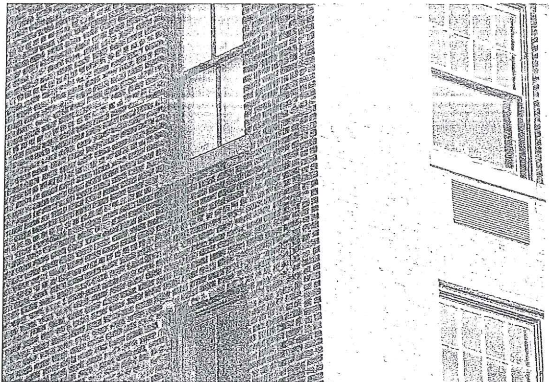
MASONRY CRACKS AT PARAPET AND WINDOW HEADS
