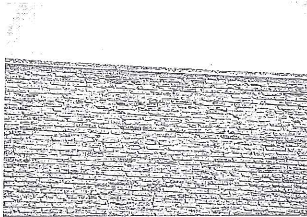
Photo 11: Spalling and erosion of the brick along the parapet at the west elevation of the Nelson House Annex. Spalling is typically evidence of freeze-thaw cycling or efflorescence – both resulting from chronic or periodic wetting of the brick. Over time, freeze-thaw cycling and efflorescence can reduce the section of the masonry wall assembly to the point where it becomes unstable.
