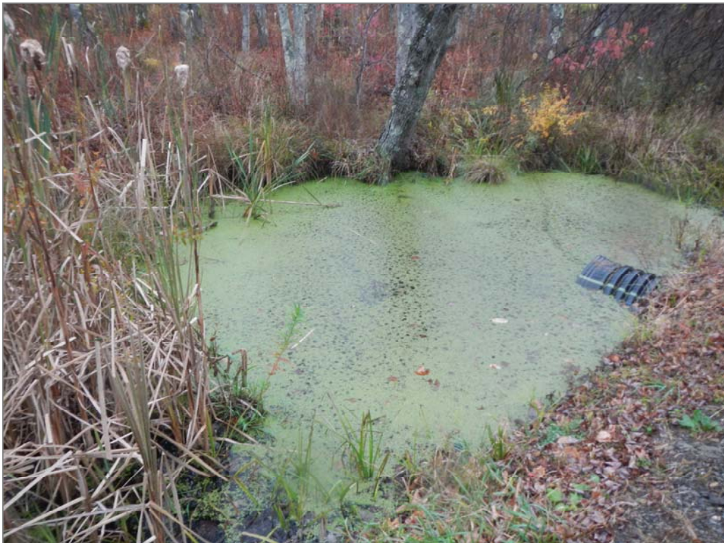
Figure 25. Some of the major culverts on Slate Quarry Rd remain unprotected by barriers, which could prevent vehicles from entering areas of standing water.
