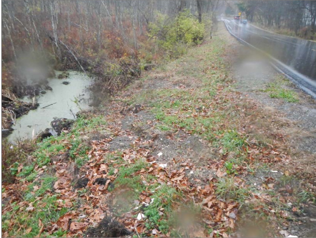
Figure 26. This area of Slate Quarry Rd may warrant guiderails to prevent vehicles from travelling into the adjacent swamp/marsh, as evidenced by the tire tracks in the shoulder.
