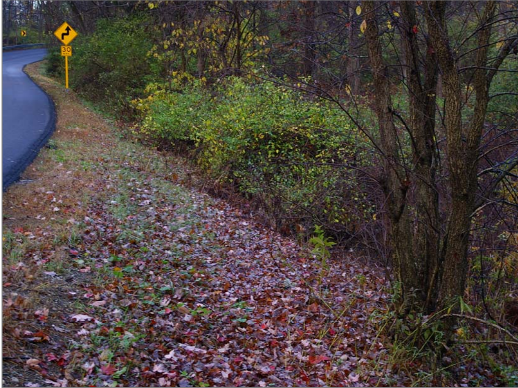
Figure 24. Sections of Slate Quarry Rd may warrant guiderails to prevent vehicles from travelling down steep embankments such as the one shown above.
