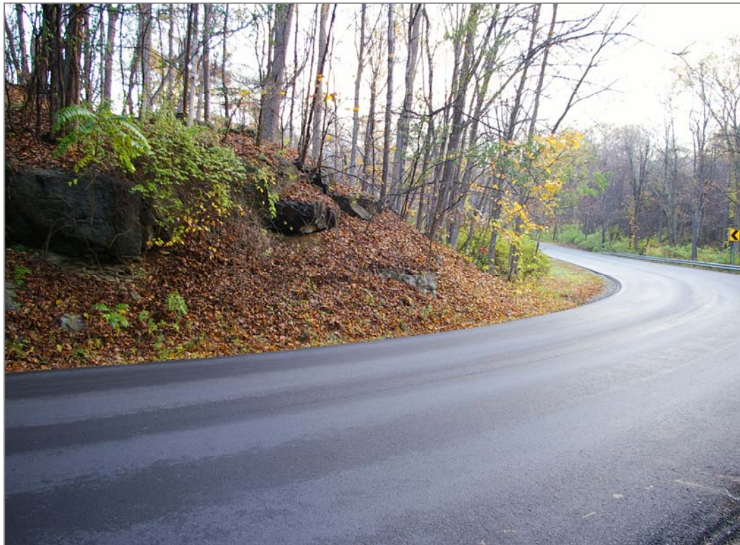
Figure 20. Looking east on Slate Quarry Rd towards the rock embankment located on the inside of the curve shown above.
