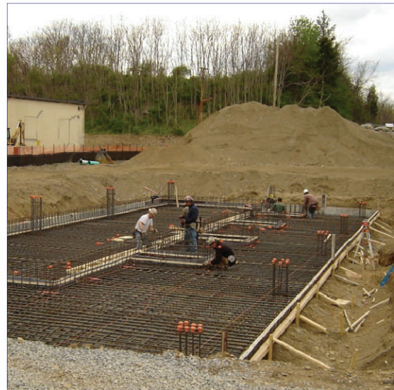
Construction of a pump station for the Central Dutchess Water Transmission Line.
