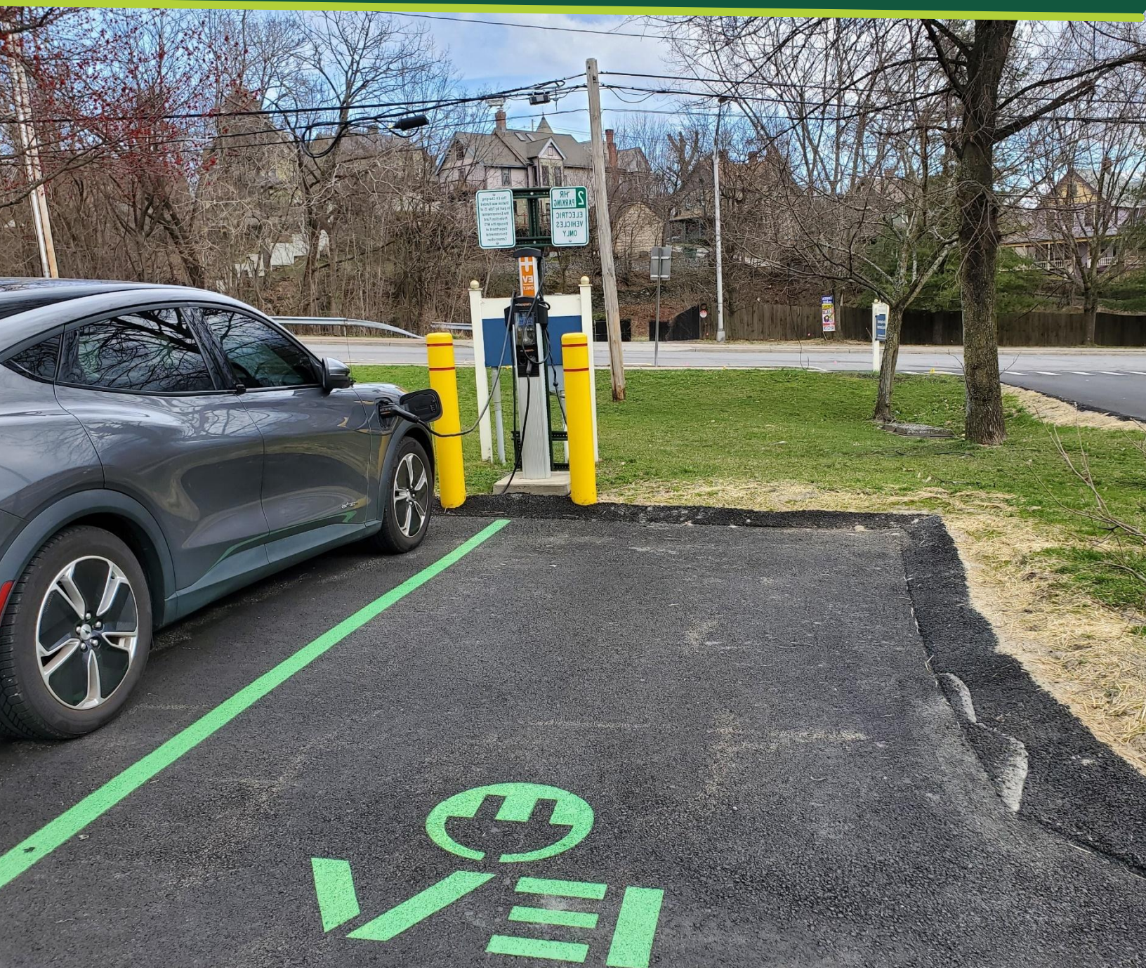
Electric vehicle using County EV charging station 2
