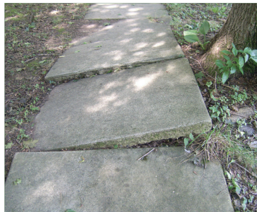
An example of lifted sidewalk pavers due to interference from tree roots.
