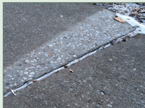
A sidewalk in the Village of Millbrook that has been shaved to even out the surface where lifting occurred.
