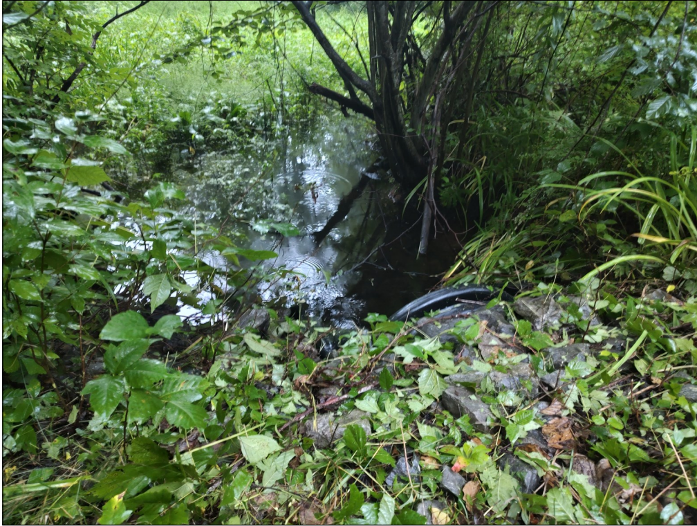
A medium-sized culvert temporarily slowing water down due to backup of flows.
