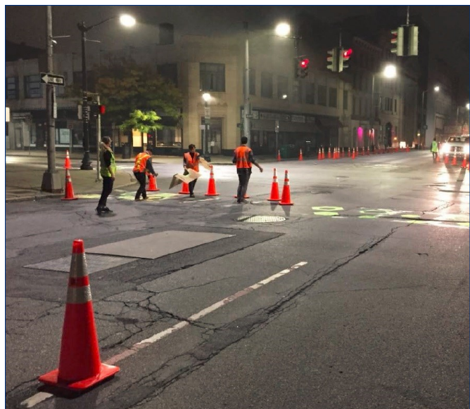
In the early morning hours, the project team worked to close a lane with traffic cones and create artistic crosswalks ahead of the morning rush hour.
