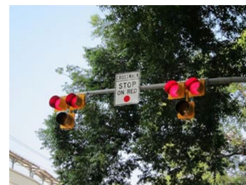
Pedestrian Hybrid Beacon (PHB) (source: FHWA)
