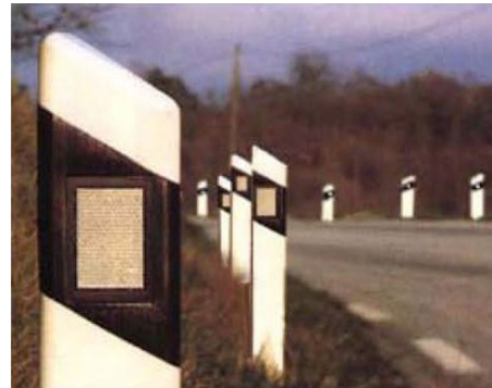
Post-mounted Delineators (source: Iowa State University Transportation Institute)
