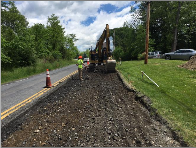
We use the TIP to program federal funds for local transportation projects such as the reconstruction of CR 9 (Beekman Rd) shown here.
