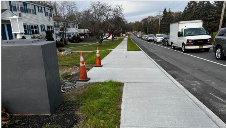
During 2023-2024, we worked with County Public Works on the scope and design of sidewalk improvements on CR 75 (Innis Ave) in the Town of Poughkeepsie.
