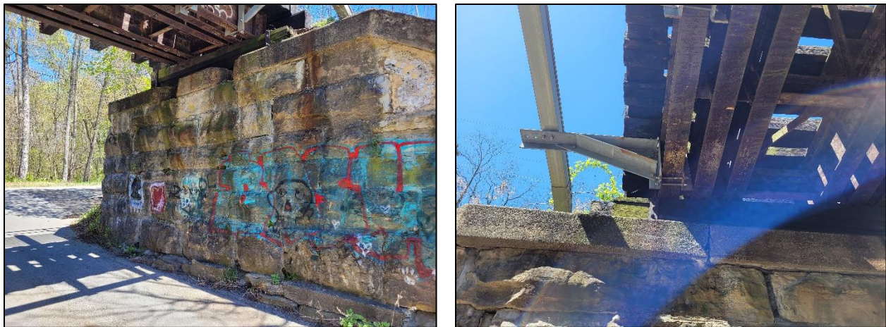
Figure 22: Bridge No. 2 concrete spalling at abutment (left) and rotated fascia girder due to utility hanger (right).
