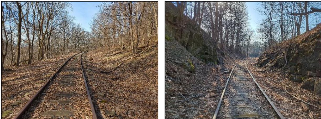
Figure 6: Defined swale on the right side of the tracks (left photo) and both sides of the tracks (right photo) with no visible signs of drainage flows.
