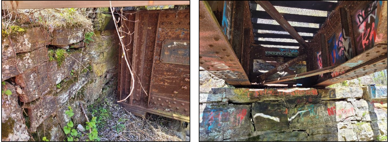
Figure 28: Bridge No. 5 west abutment backwall – missing mortar (left) and east abutment stem – missing mortar (right).
