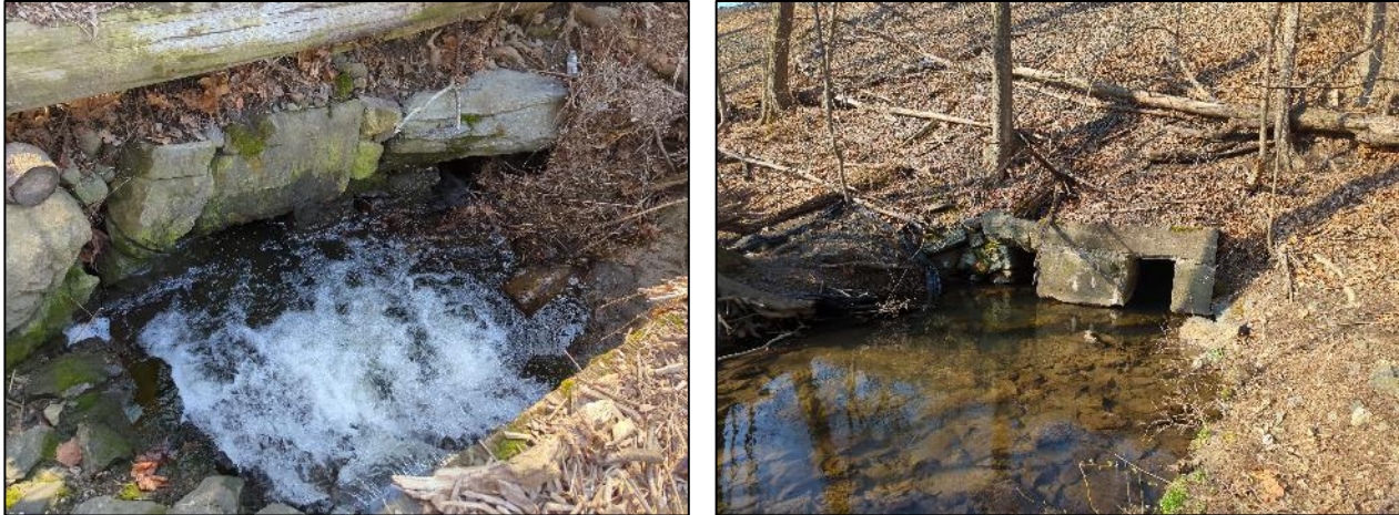
Figure 4: Blocked inlet of double barrel stone culvert surrounded by wooden debris (left) and outlet of double barrel stone culvert flowing under railroad (right).
