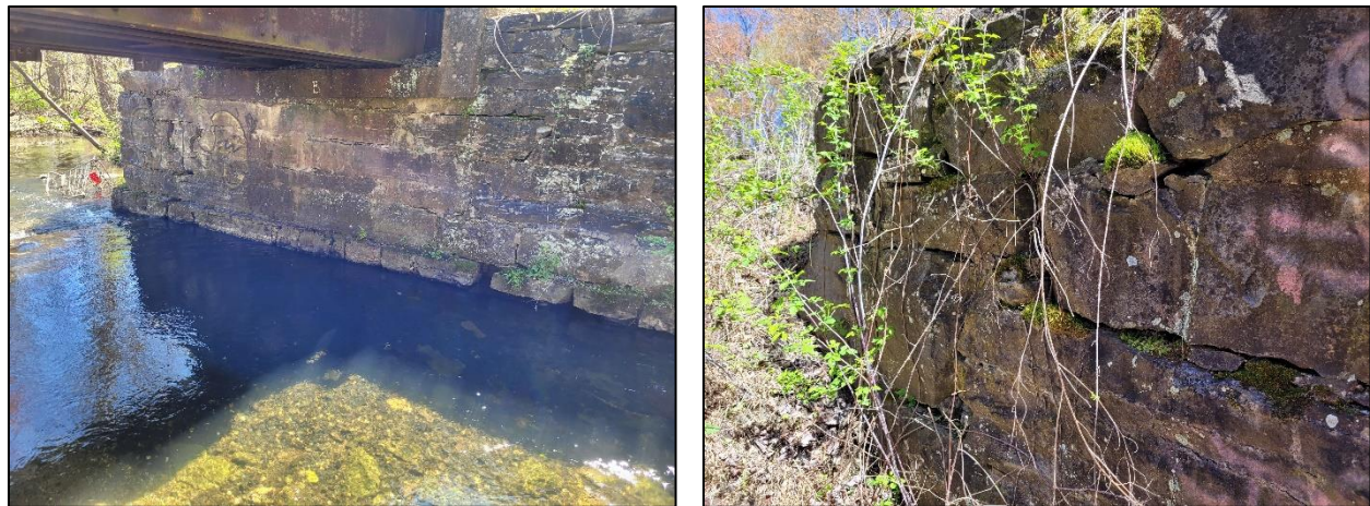
Figure 30: Bridge No. 6 west abutment – void in footing stone (left) and east abutment – missing mortar (right).
