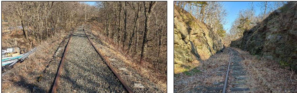
Figure 13: Steep fill slopes and a narrow railroad corridor (left) and rock cut and narrow railroad corridor (right).
