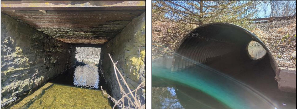
Figure 3: Stacked stone culvert with steel railroad rail top slab (left) and inlet of 9-foot-wide corrugated steel three-sided arch structure (right).
