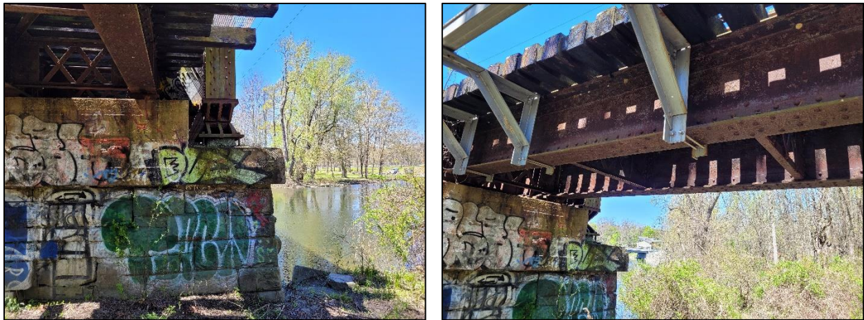
Figure 26: Bridge No. 4 pier 2 rotated stones (left) and surface corrosion at steel girders (right).
