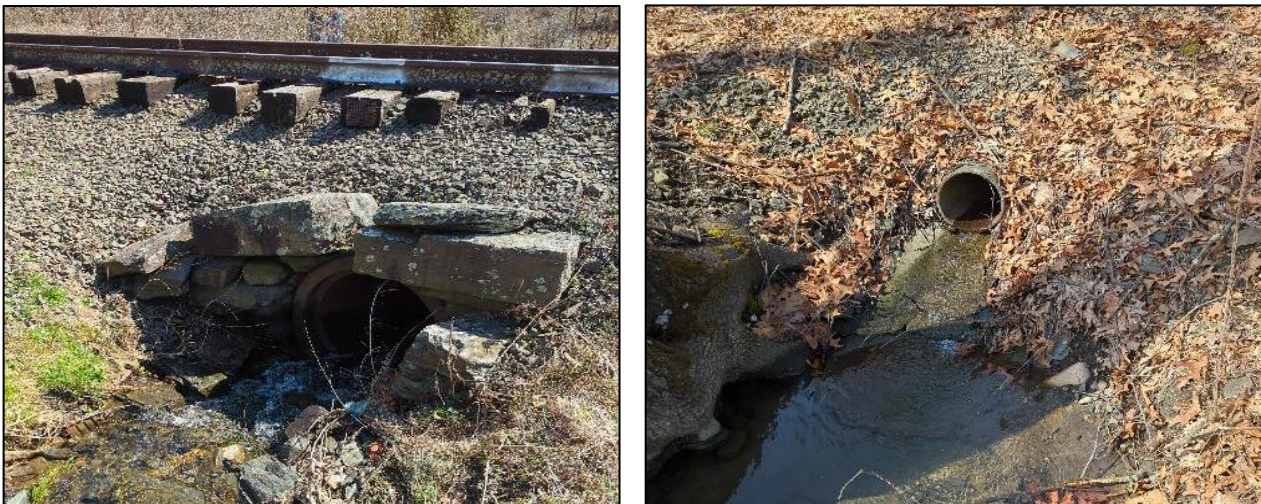
Figure 5: Small smooth steel culvert pipes representative of those found throughout the corridor.
