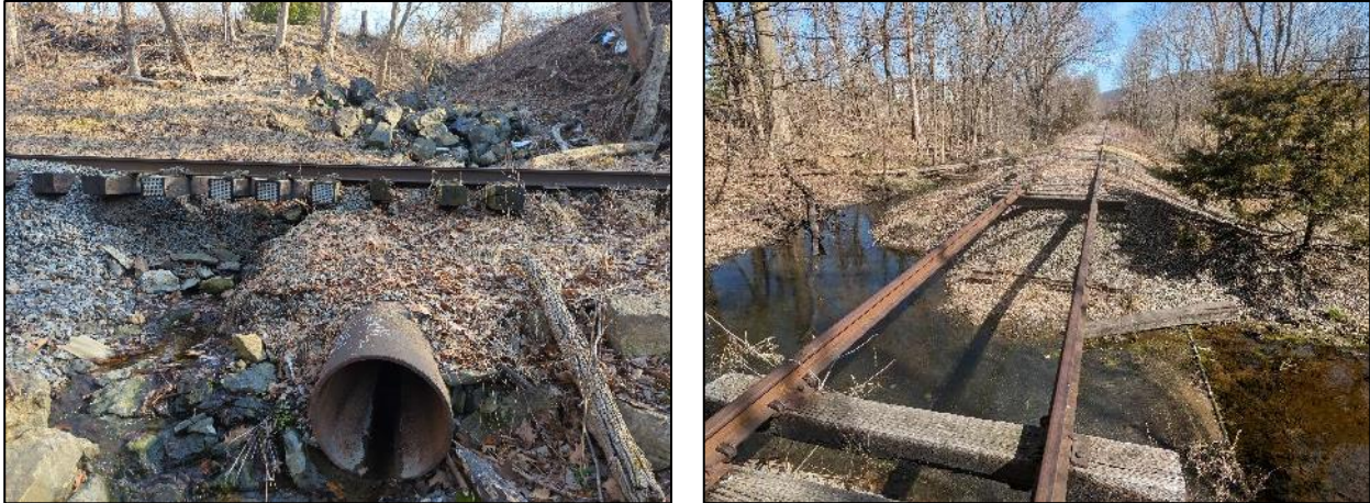
Figure 7: Washout 0.25 miles west of Washington Ave (left) and large washout 0.20 miles east of Route 9 (right).
